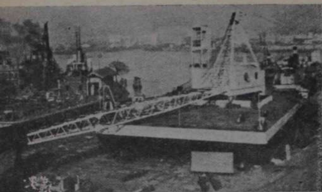
Barcaza para transportar nafta y grúa flotante de 30 toneladas, en transformación y montaje, en el Astillero Central del Ministerio de Obras Públicas a lighter for the transport of naphtha and a floating crane of 30 tons, seen during the process of its transformation and assembly in the Central shipyard of the Ministry of Public Works
